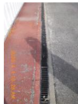
Chemicals warehouse spill retention system.JPG
